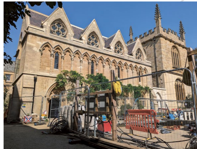
THE STONEMWORK OF THE LIBRARY HAS BEEN REPAIRED, BUT THE MOST NOTICEABLE CHANGE IS THE CREATION OF A NEW ENTRANCE, NEXT TO THE BODLEIAN
