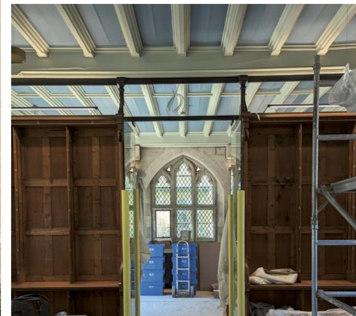
THE CEILING OF THE GROUND FLOOR HAS BEEN PAINTED AN UNDERSTATED DUSTY BLUE
